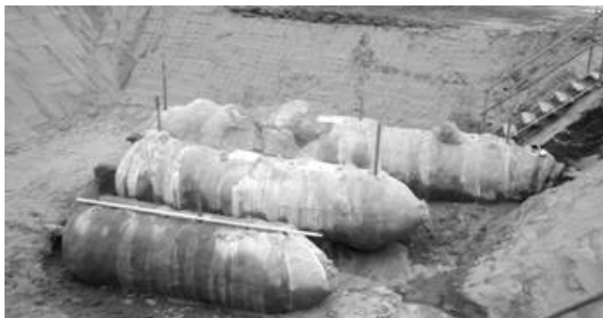
Figure 8. Horizontally laid jet-grouted columns at the test site in Tokai after excavation.
